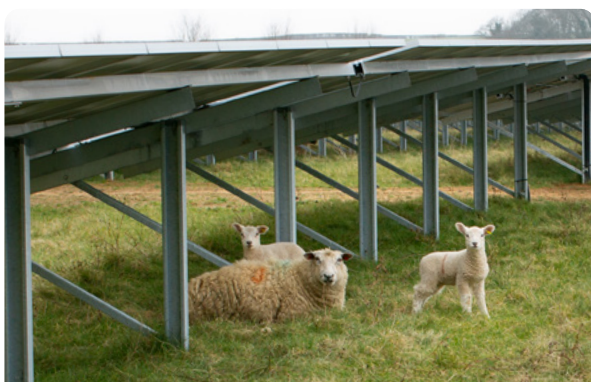
Solar PV modules mounted onto arrays
