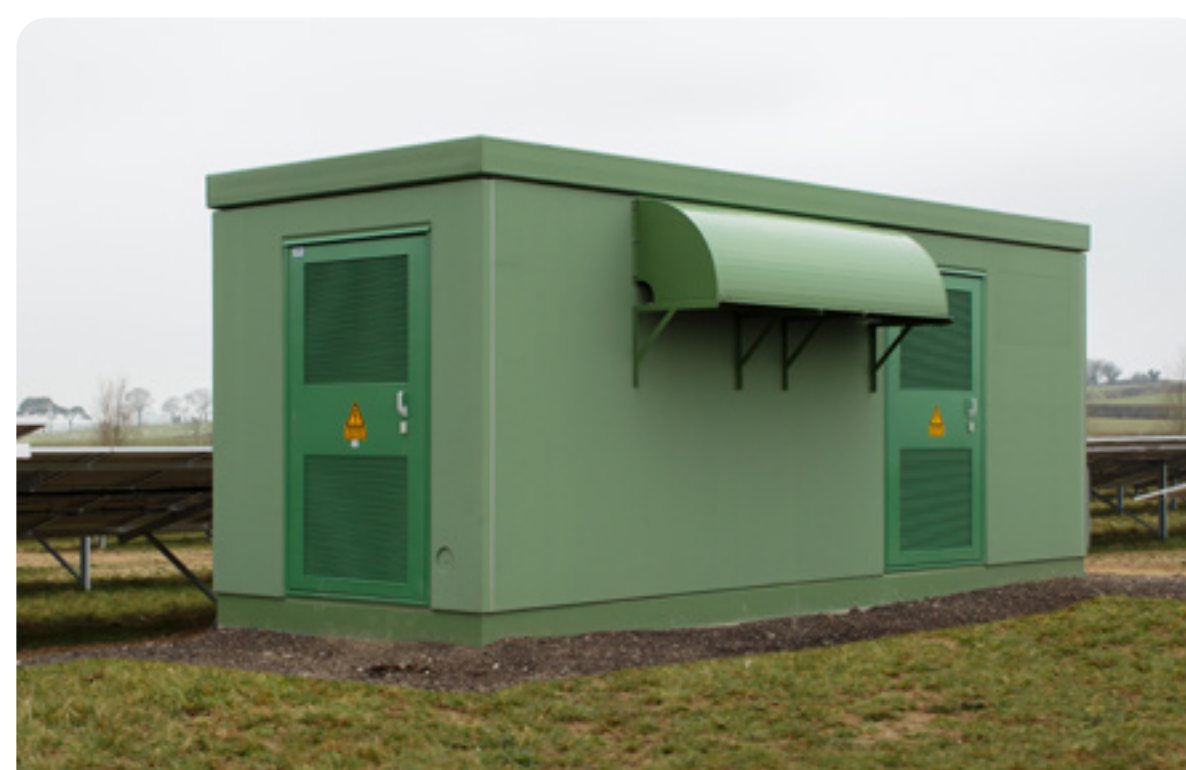
Inverter / transformer units
